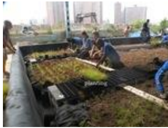
BCEQ created a popup wetland to clean the water from the highway before it reached the river.
