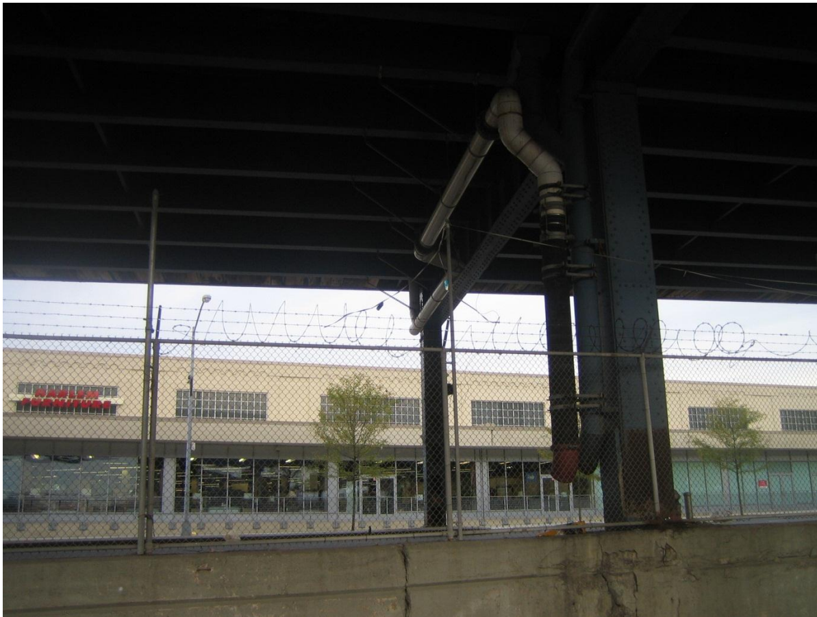
Pipes go from both the northbound and southbound side of the highway.
