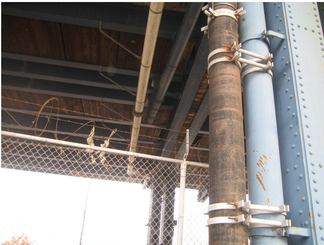
Another view of the runoff piped onto the future parkland.
