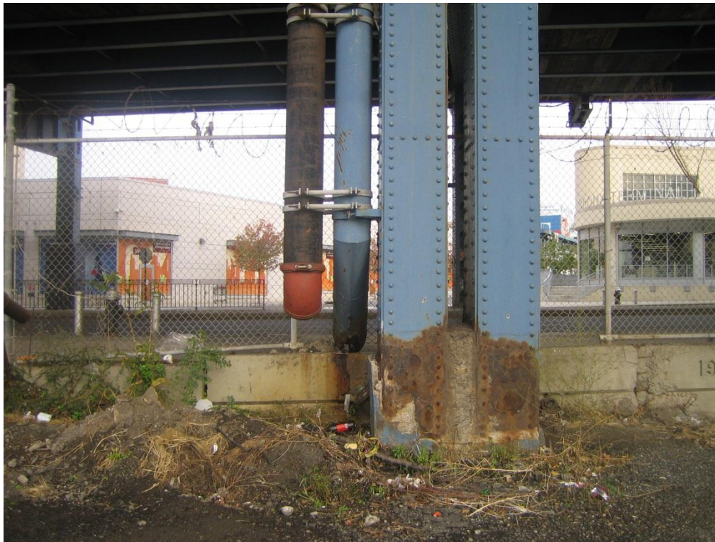
Both sides of the runoff from the elevated highway land on the future parkland.
