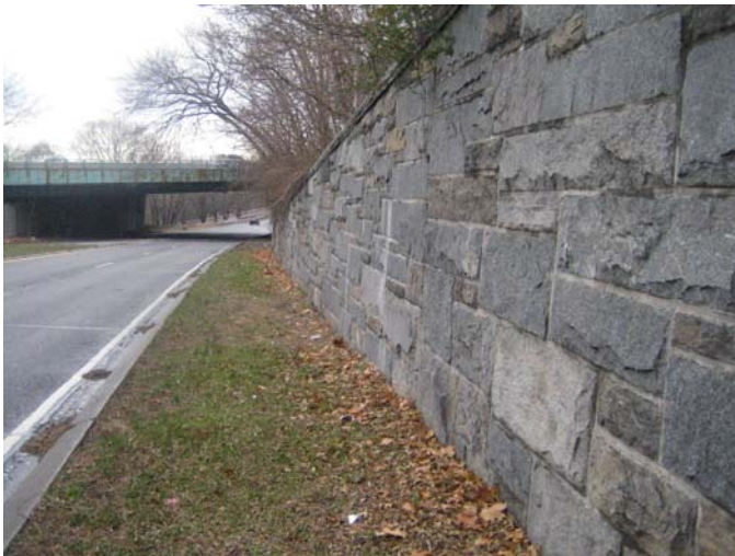
View of the retaining wall and the Mosholu Underpass (Major Deegan Expressway Overpass, looking north)
