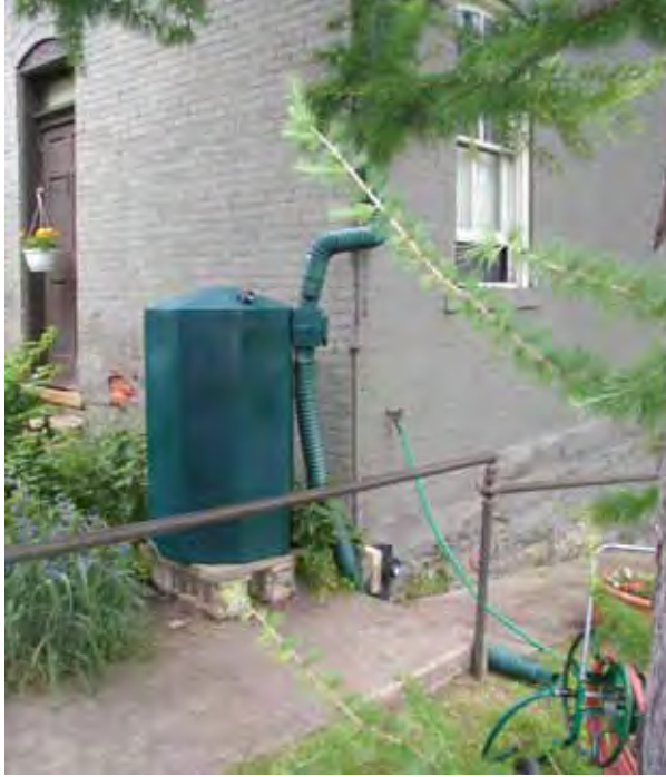
A RiverSafe RainBarrel installed at the Jane Holmes nursing residence in Pittsburgh, PA, by the Nine Mile Run RainBarrel Initiative.
